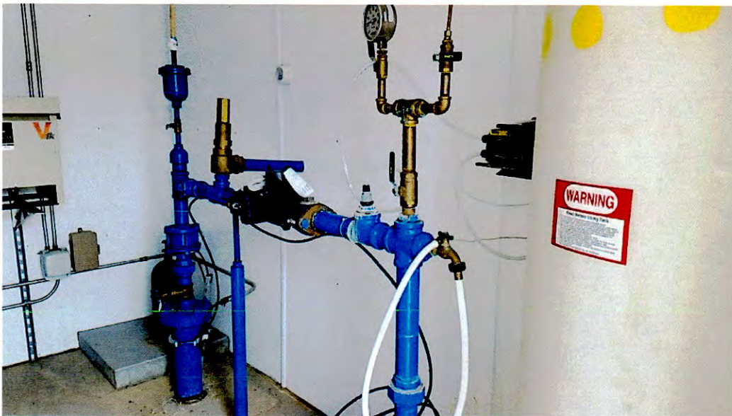
Manifold installation in well house
