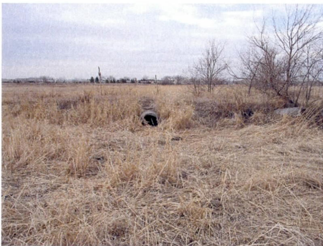
Pipe at Reservoir
