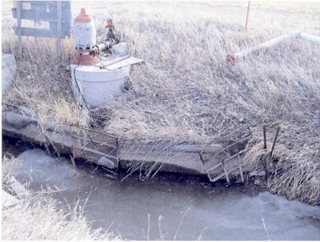
Northeast Pump and Intakes
