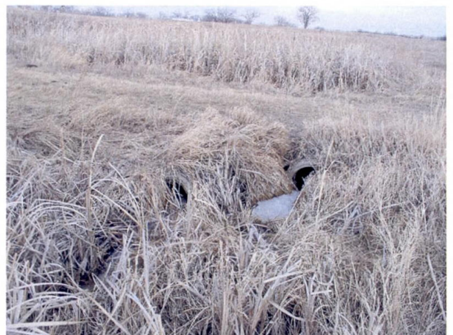
Pipe at Reservoir
