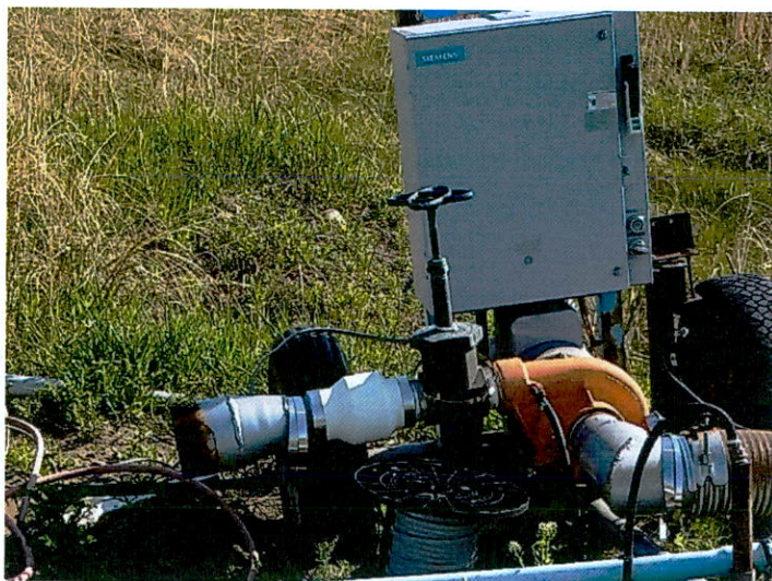
Pump for center pivot
