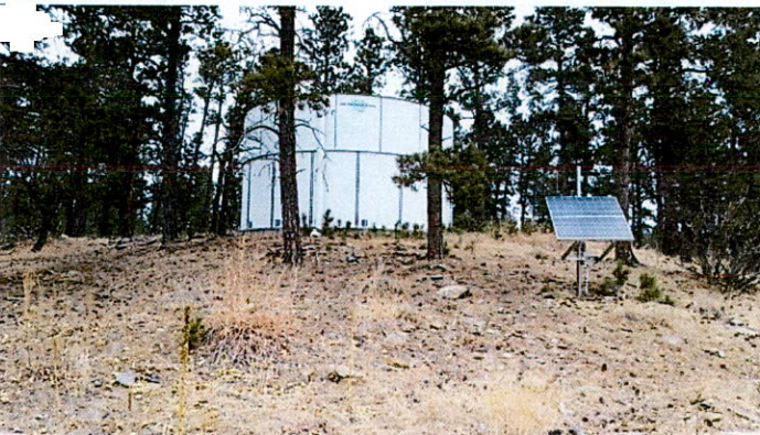
60,000 gallon Storage Reservoir
