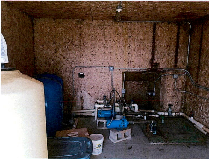
pump house appurtenances
