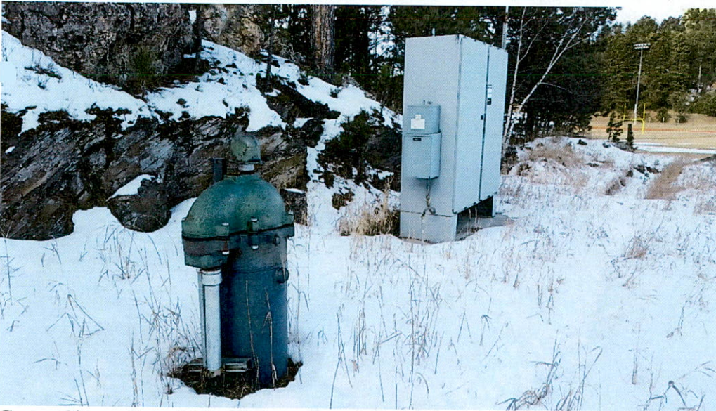
Custer City well no. 11 located southeast of athletic field
