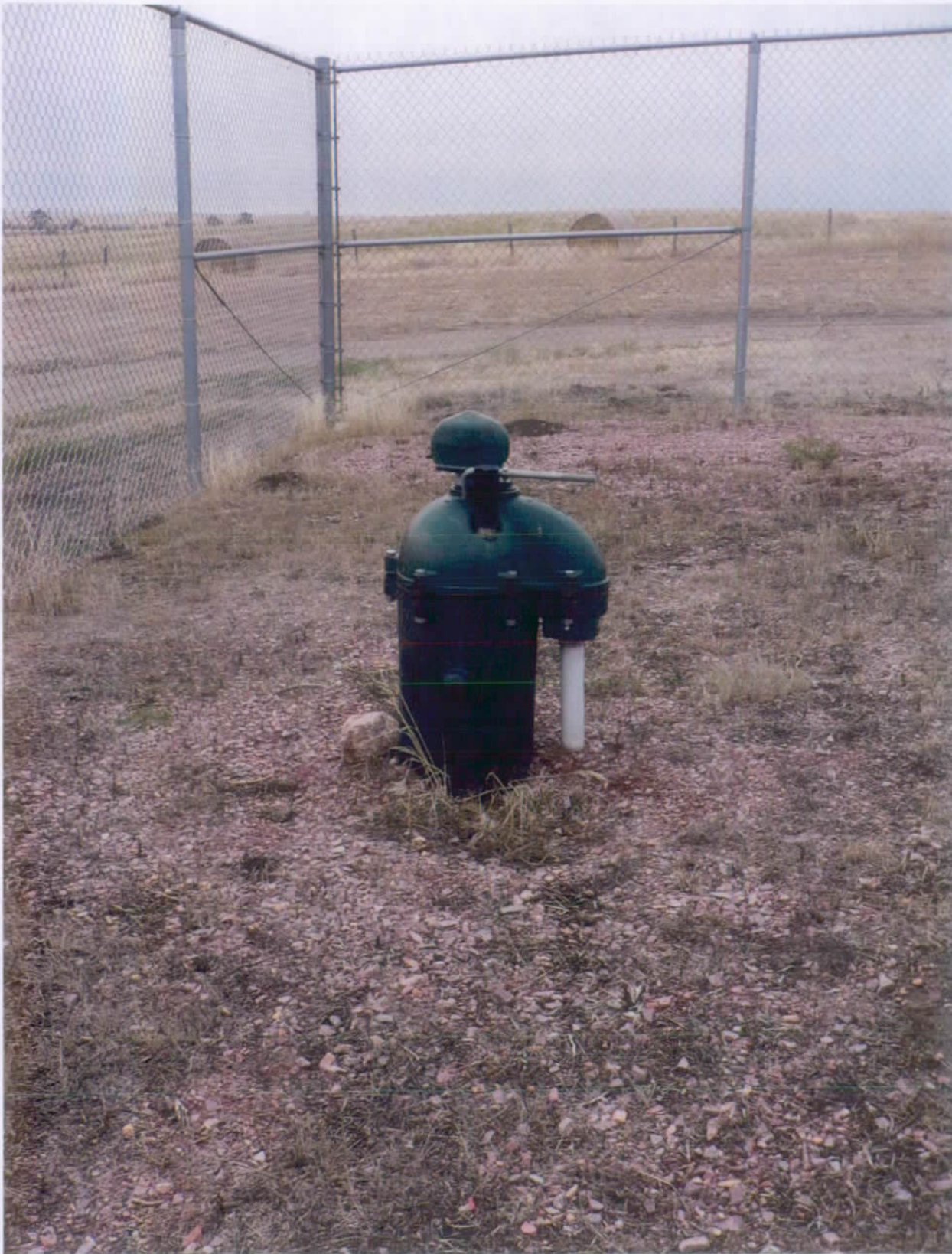
City of Martin Well No. 5 authorized by Water Permit No. 2517-2
