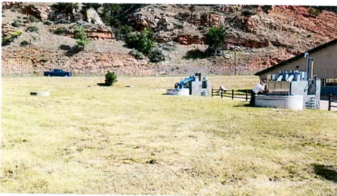
Area of collection gallery and rearing pavilion pumps
