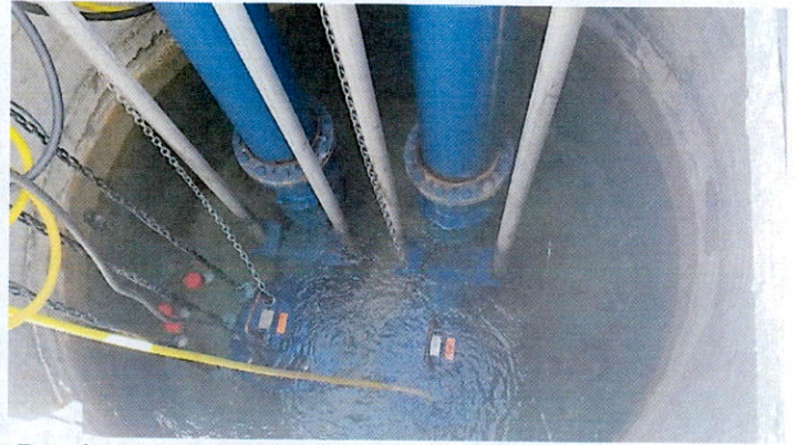
Rearing pavilion pumps
