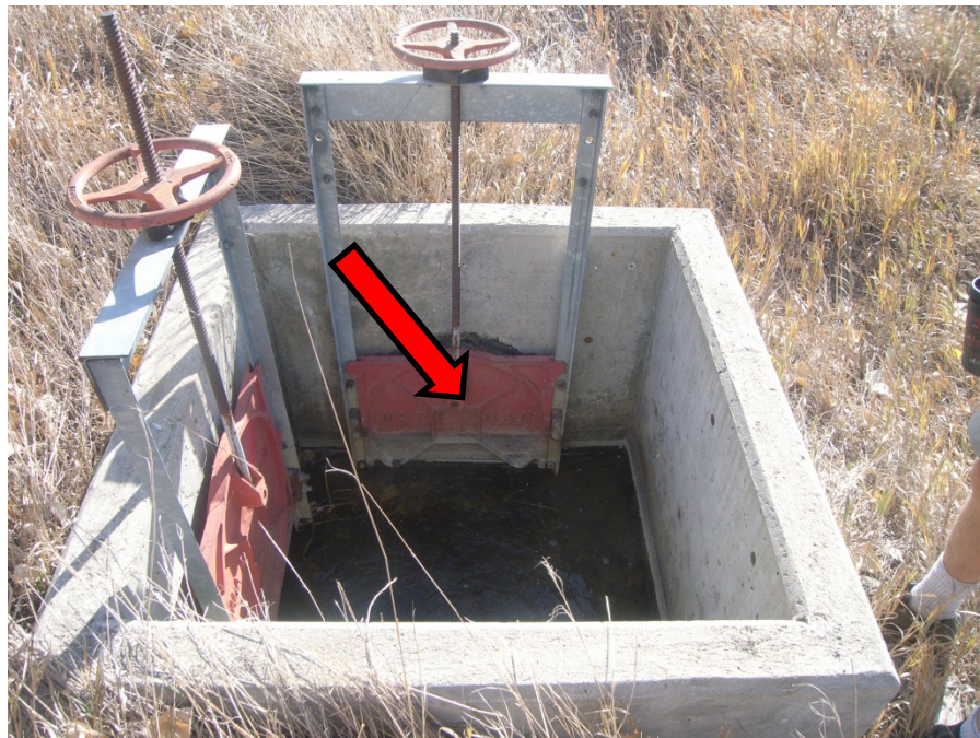
Figure 3-20. Junction Box With 24-Inch Canal Gate for Turnout C of Permit 2512-2 (Turnout C Shown With Red Arrow, Leading South).
