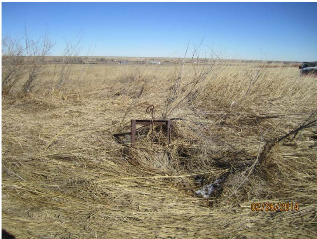
Figure 3-33. Metal Framed Canal Gate of Turnout D Associated With Permit 2249-2.
