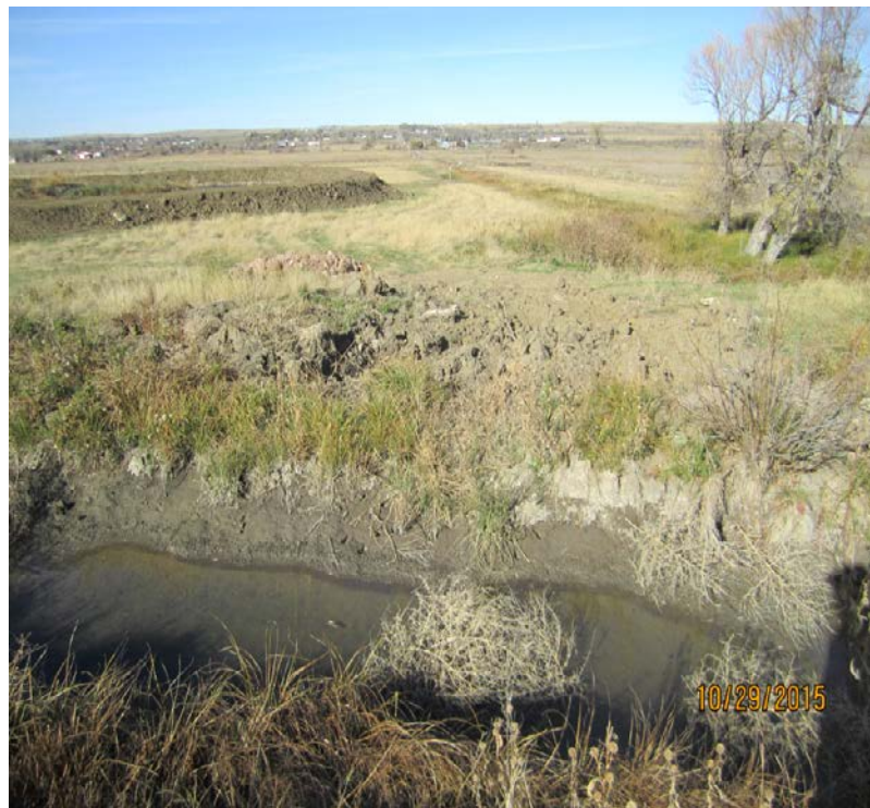
Figure 3-36. Turnout B Associated with Permit 2249-2. The old turnout structure has been removed. Date 10/29/2015.
