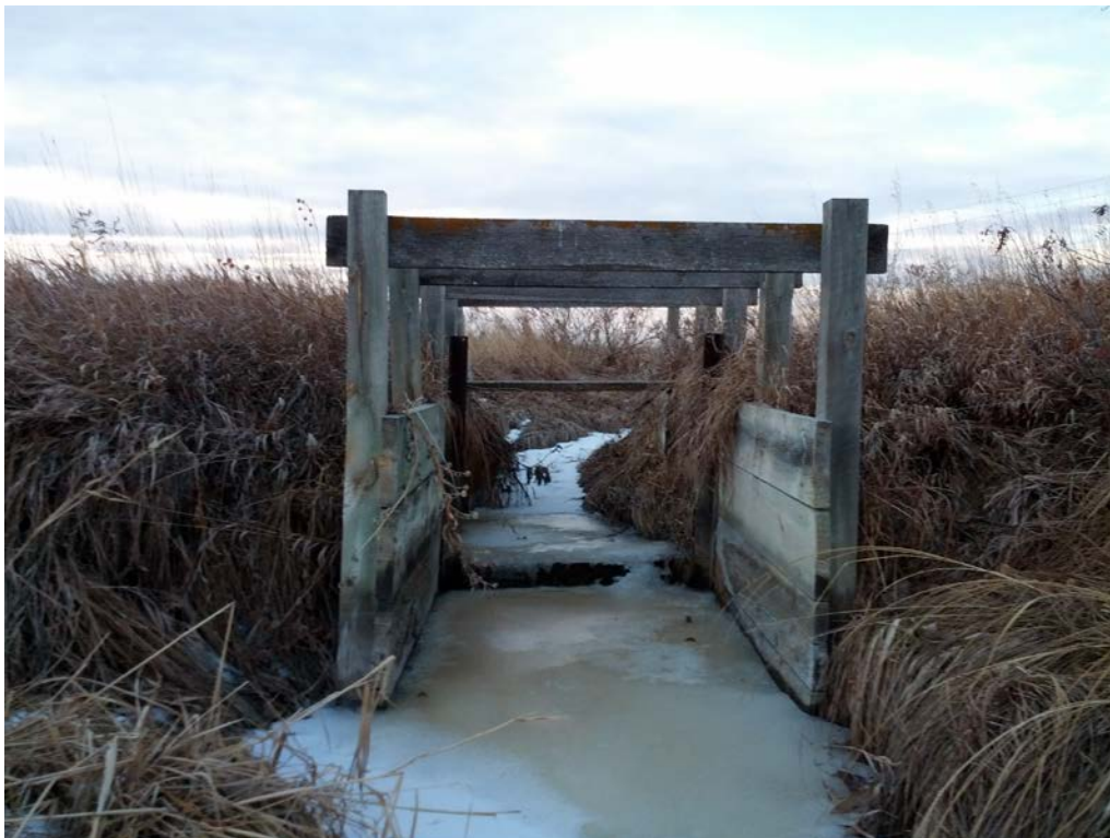
Figure 3-43. Wooden Flume Used as a Check for Turnout A of Permit 2415-2.
