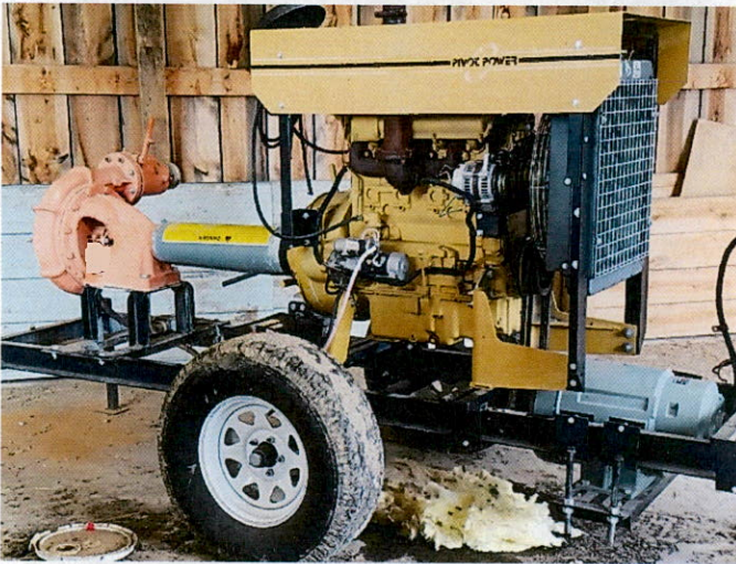
Diesel pump and generator
