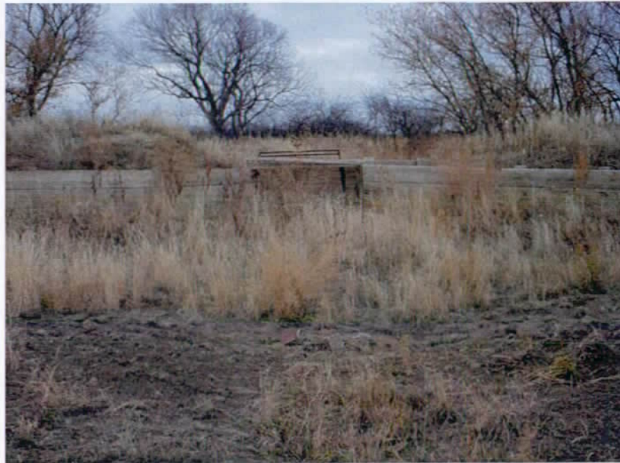
Picture of diversion structure. If gates are open flow from Dirty Womans Draw enters an irrigation ditch which supplies the water for spreading
