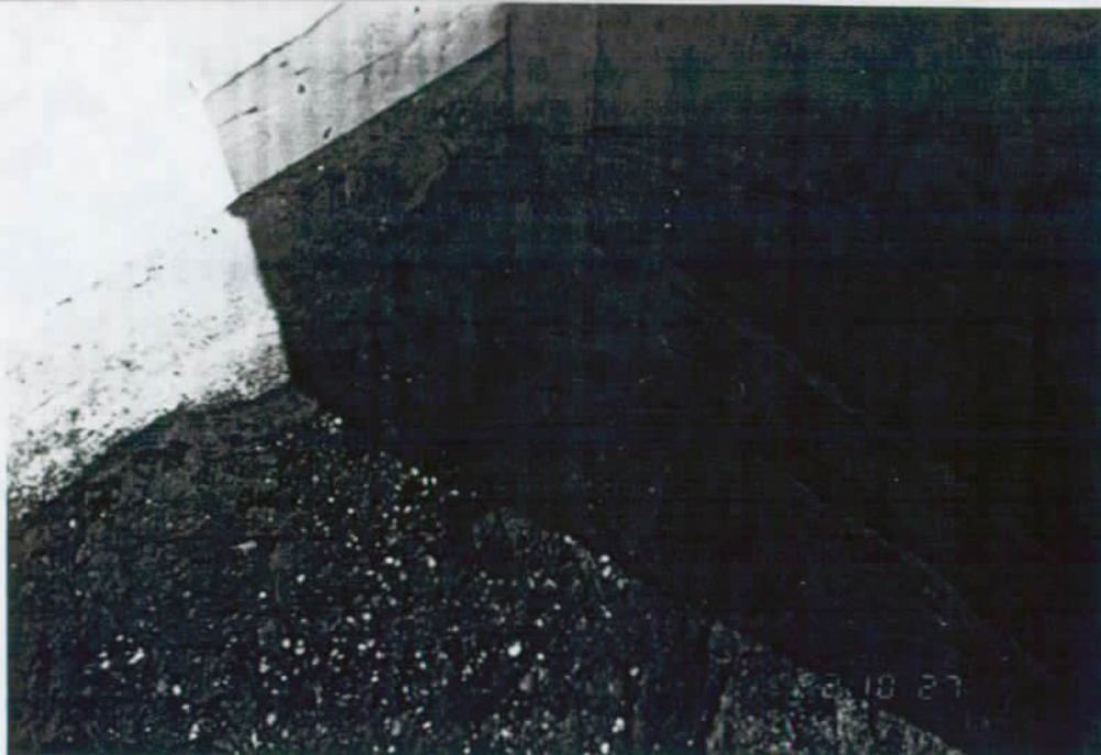
PHOTO NO. 9 MAYO I RODENT /RUNOFF UNDERMINING OF SLAB
