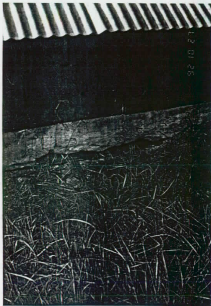
PHOTO NO. 12 DETERIORATED SPRING VAULT AT MAYO DEEP WELL
