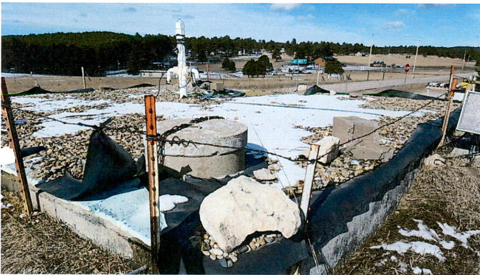
20,000 gallon storage reservoir
