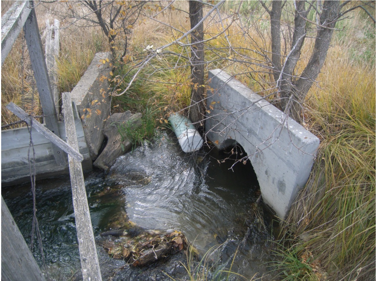
Figure 3-7. Pipe Turnout B for Permit 2469-2.
