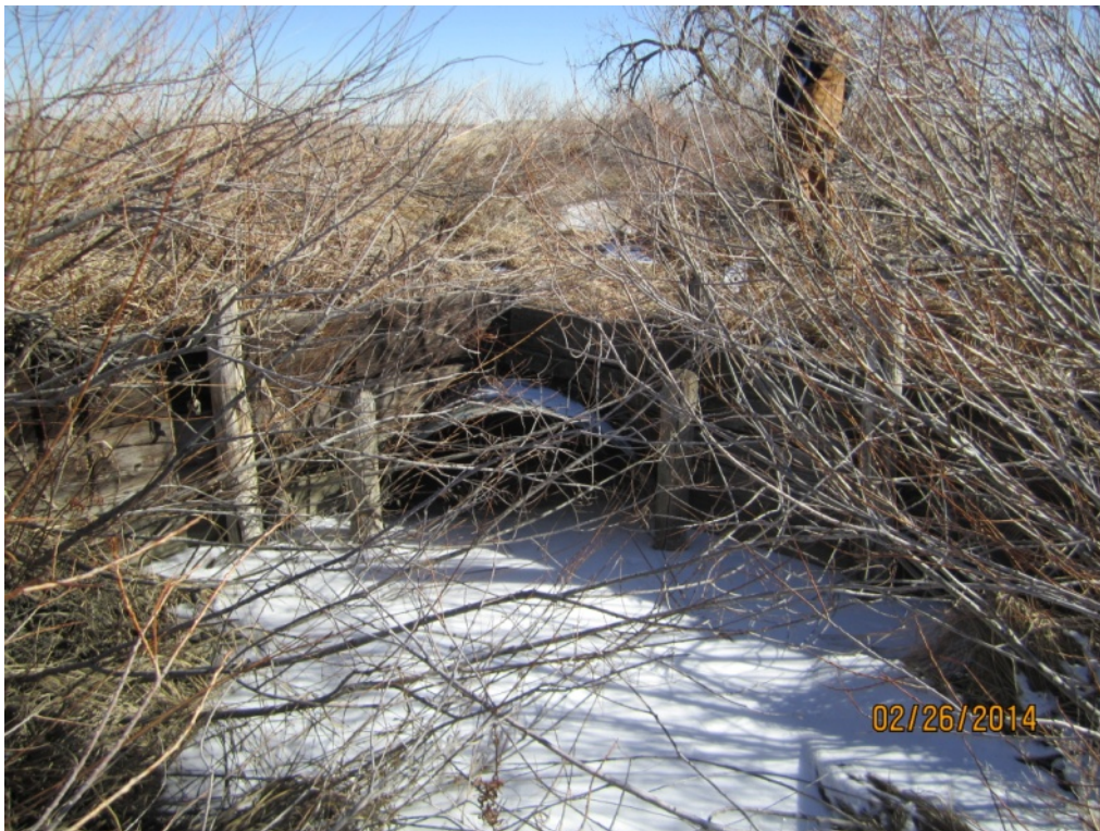
Figure 3-31. Second Culvert Crossing, Used as Check for Turnout C Associated With Permit 2249-2.
