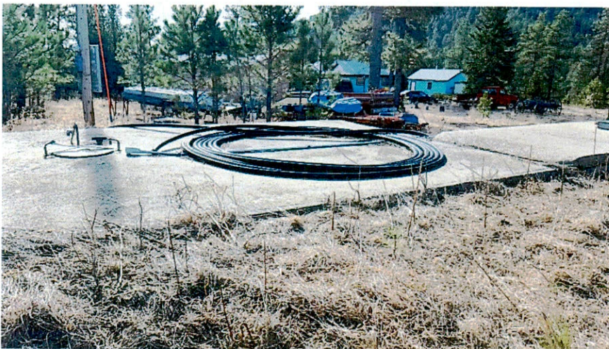
Cistern and booster station
