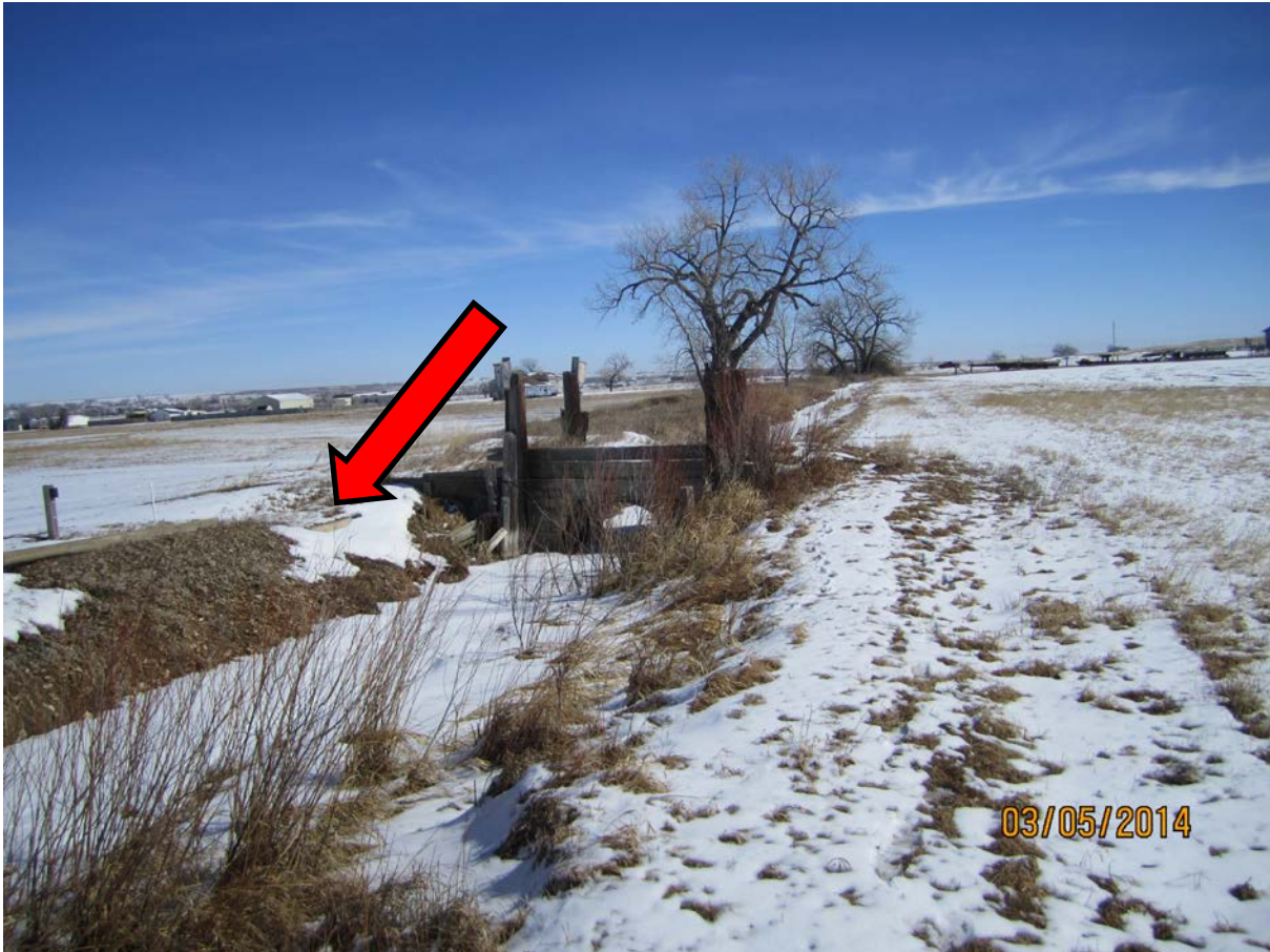
Figure 3-23. Turnout for Permit 2234-2. Note the headwall sticking out of the snow just upstream from the culvert crossing on the left or north side of the ditch (red arrow). The ditch behind the headwall has been filled in.
