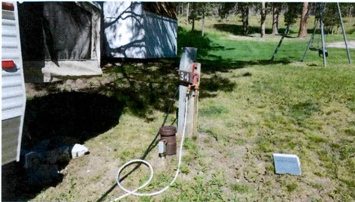
Well # 1 (temporarily abandoned)
