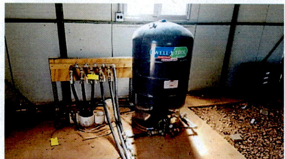
Pump house appurtenances
