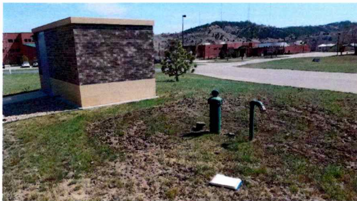
Well and pump house
