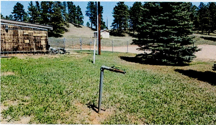
System outlet with well in background
