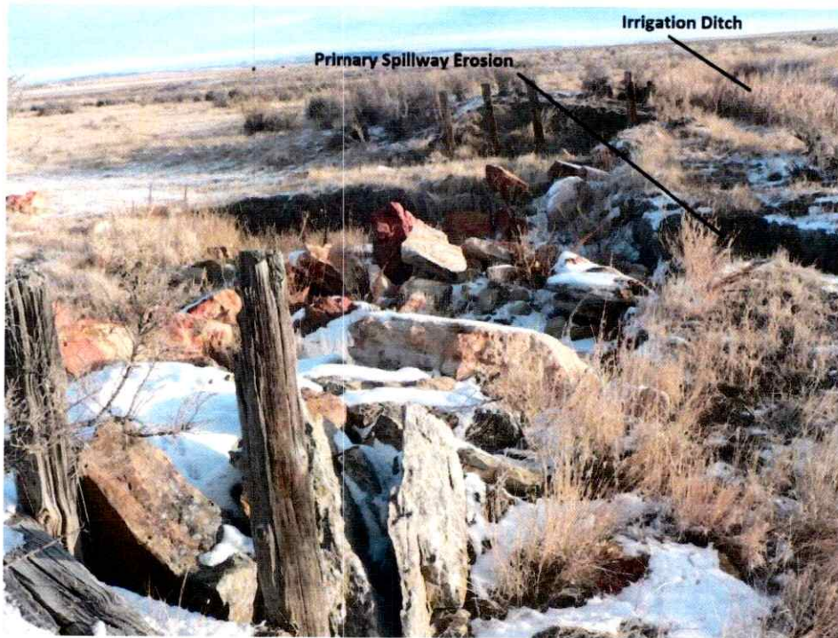
Figure 4 – Photo showing a side view of the downcutting erosion of the primary spillway with the irrigation ditch off to the right.
