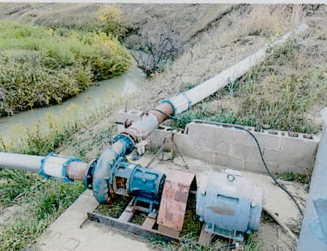
diversion point downstream of storage
