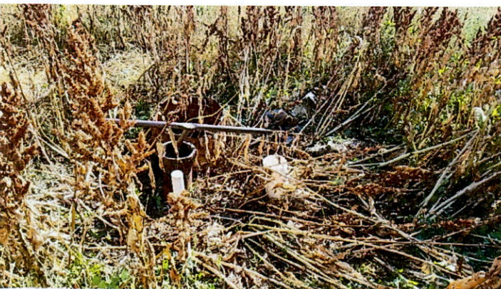
6" Irrigation outlet from 18" effluent line
