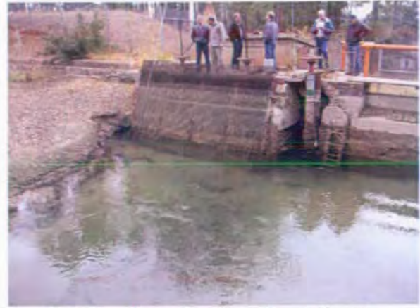
Forebay Dam. Outflow Trash Grates
