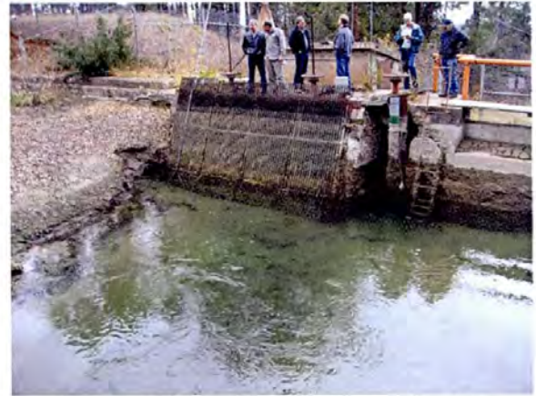
Forebay Dam. Outflow Trash Grates
