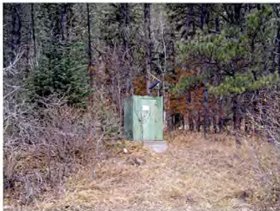
USGS Maurice Gage. Data Transmitter Site
