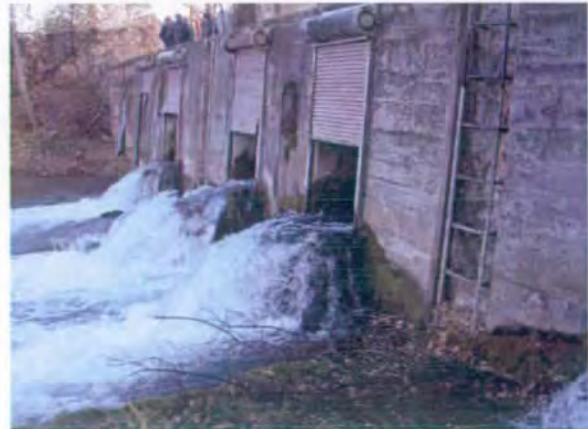
Powerhouse. Water Return
