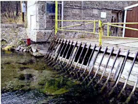
Maurice Dam. Diversion Grates
