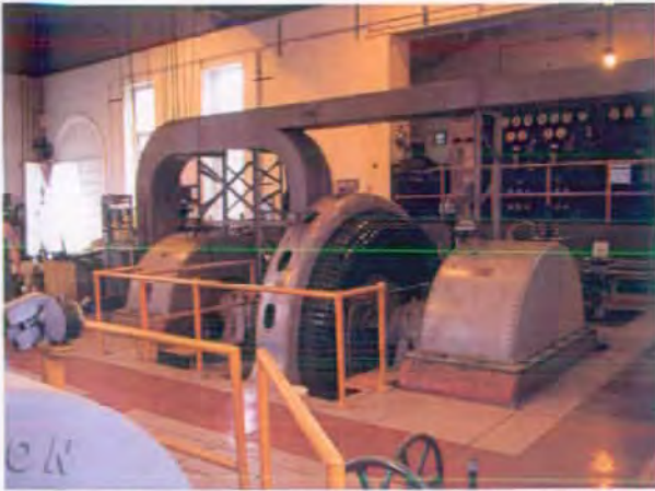
Powerhouse. Generator and Pelton Wheels
