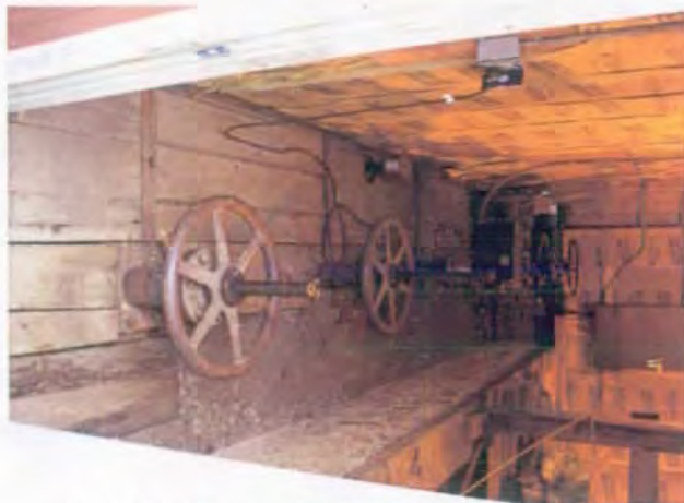
Maurice Dam. Diversion Gate Controls
