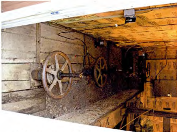
Maurice Dam. Diversion Gate Controls
