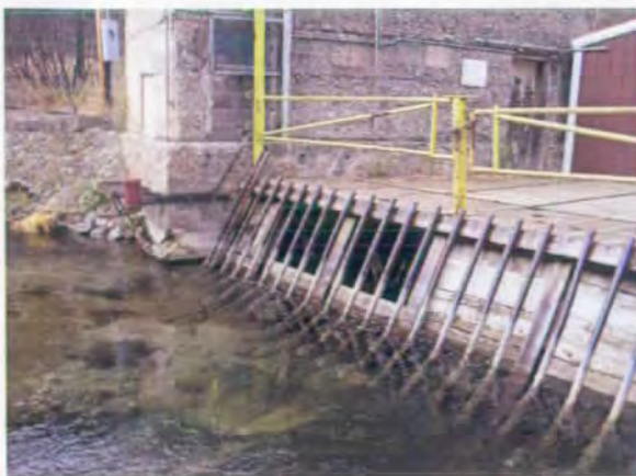
Maurice Dam. Diversion Grates
