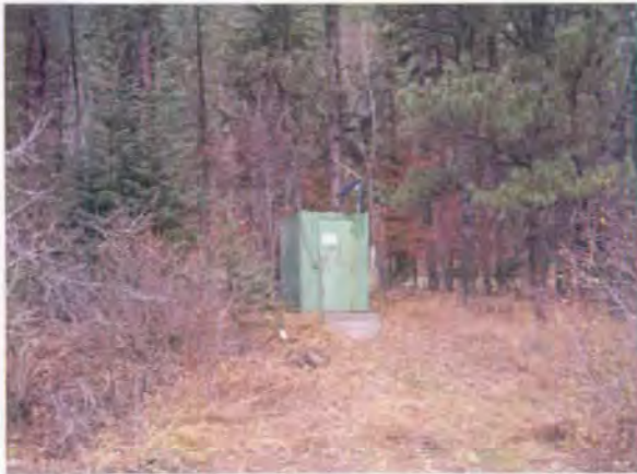
USGS Maurice Gage. Data Transmitter Site
