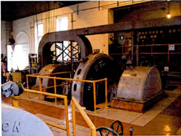
Powerhouse. Generator and Pelton Wheels
