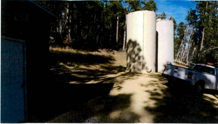
Twin 25,000 gal. storage with well house in foreground
