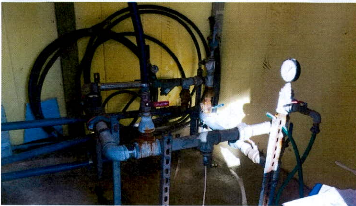
Pump house manifold
