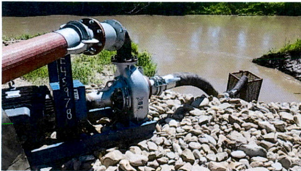
Belle Fourche river diversion pump
