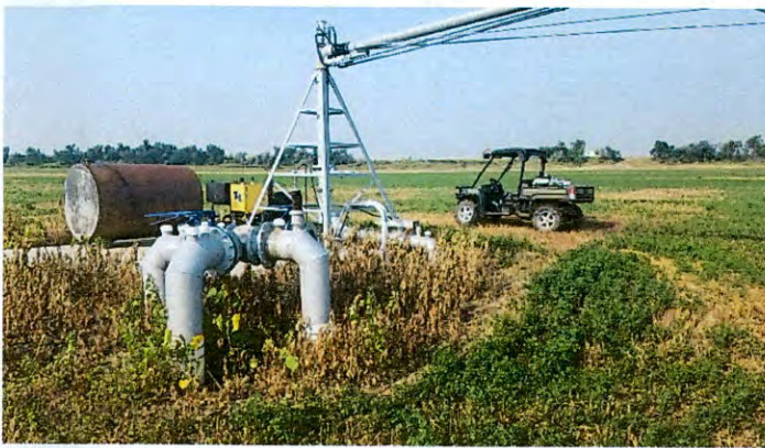
Supply line from river and manifold piping to each of the three pivots (in foreground) at No. 2 pivot
