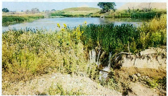
Belle Fourche Irrigation District wasteway pond with embankment washed out. This was the supply source for gravity irrigation when the acreage was supplied by the Irrigation District. The pond is no longer used for irrigation supply.
