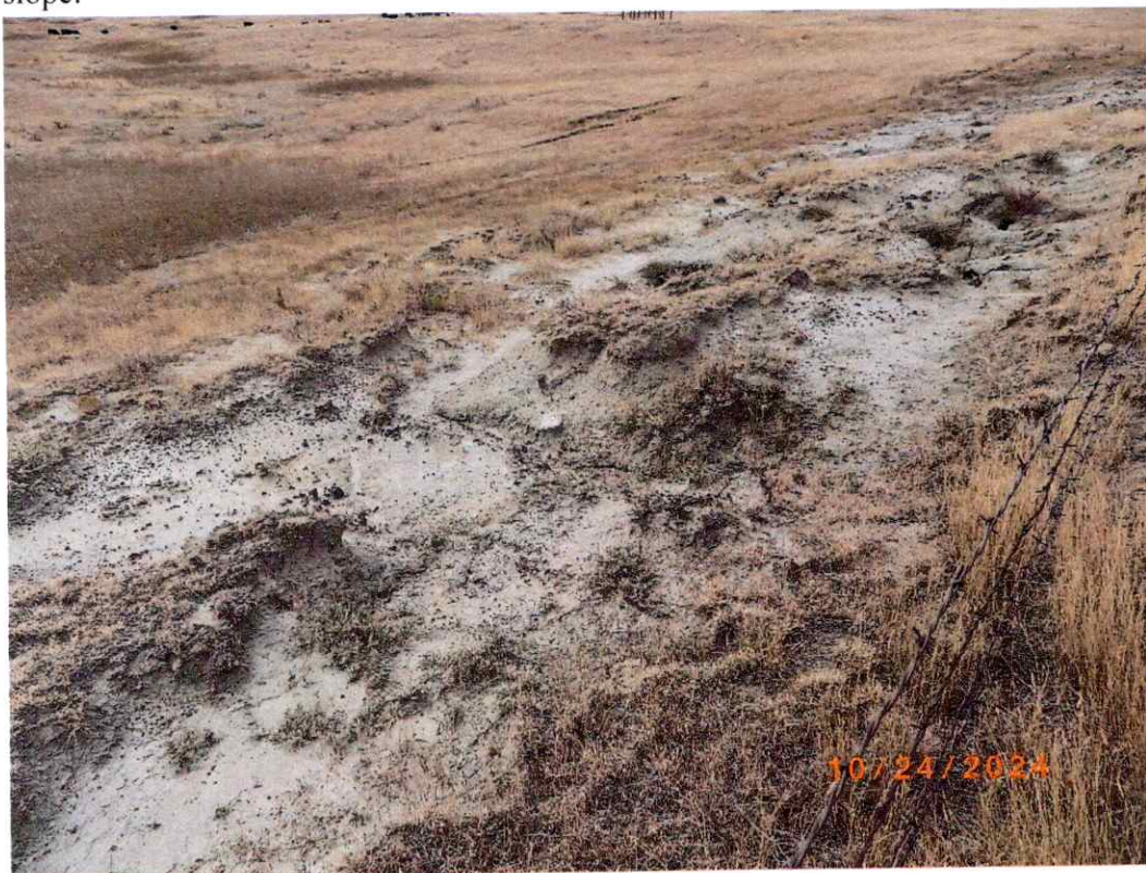
Example of inadequate grass cover and erosion of the lower right side of the downstream slope.
