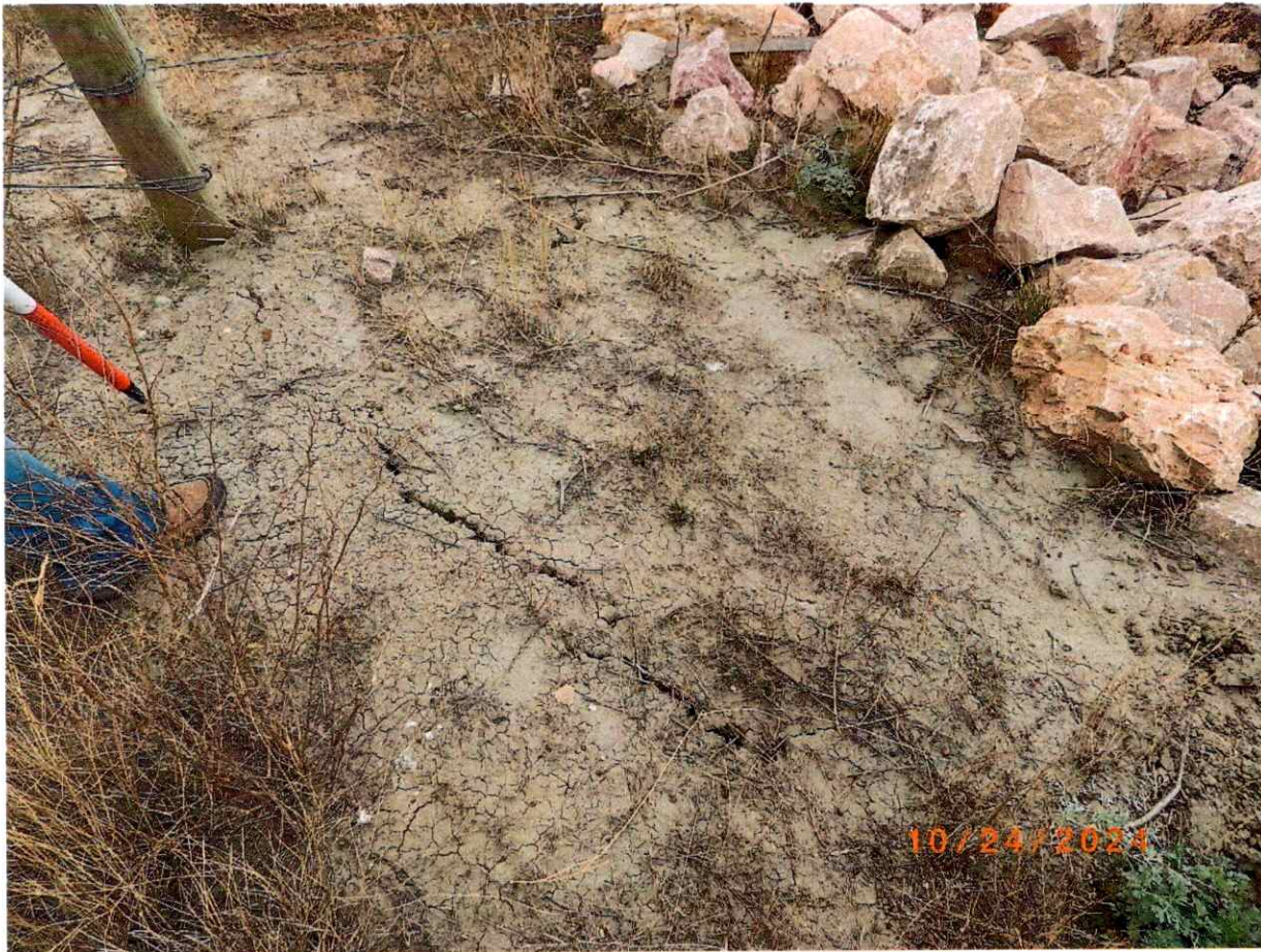
Example of cracking on downstream slope.
