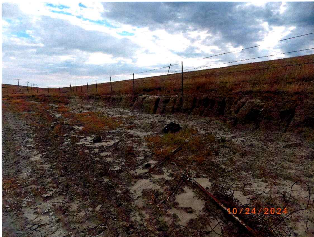
Upstream slope, note extensive erosion and proximate to fence line.
