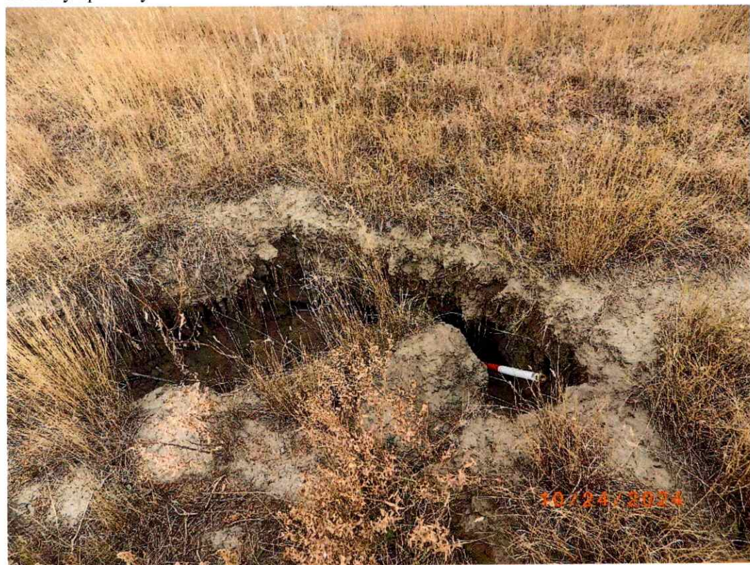
Downstream slope sinkhole right side of dam near fence. Survey rod picture is 4ft long.
