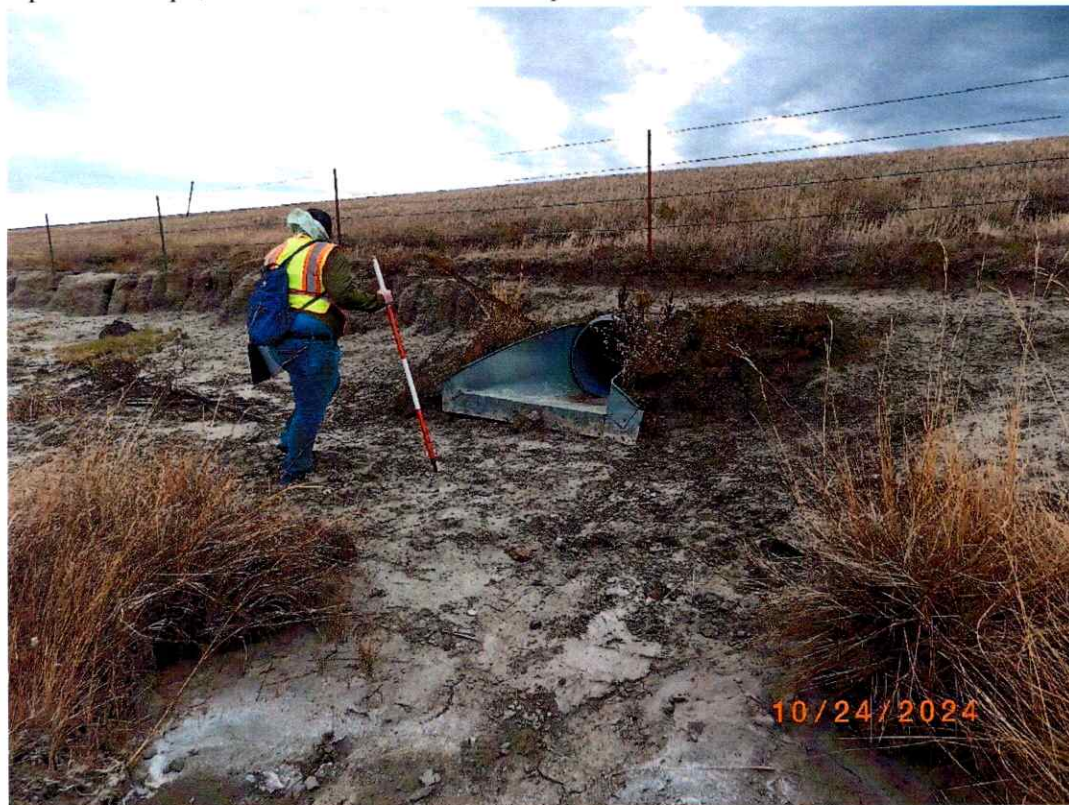
Erosion line in relation to inlet. Note erosion area are present above conduit and older erosion above fence line and lack of riprap and grass cover.
