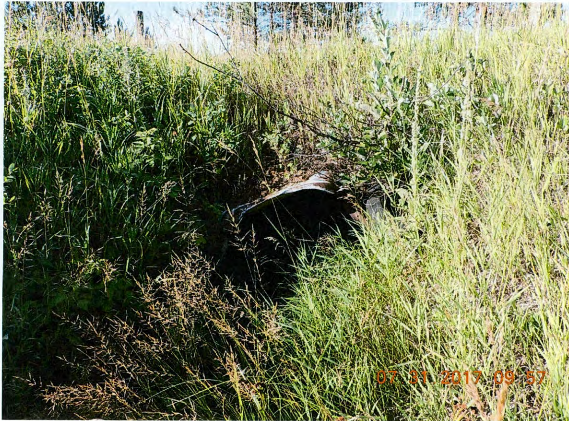
Pond #2 - 4' diameter corrugated metal pipe serving as secondary spillway.
