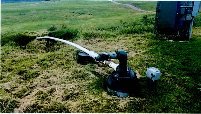
Well and piping to ponds
