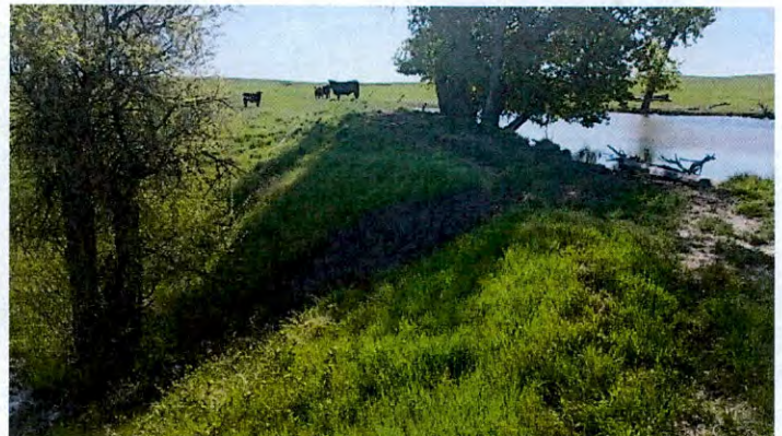
Showing downstream slope erosion from west abutment
