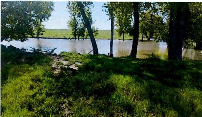
Showing pool from west abutment, water level within 1' of overtopping dam.
