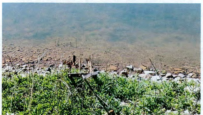
Old head gate with hand wheel deteriorated and bent over
