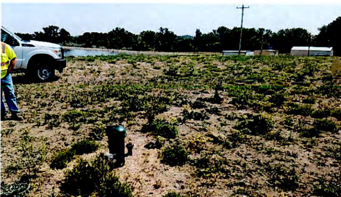
Well head with water treatment plant in background
