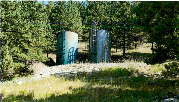
Twin 20,000 gallon steel storage
