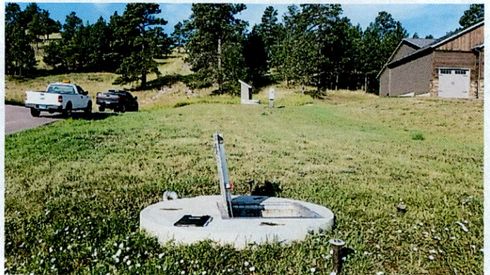
Booster pit for lower system with well pit in background
