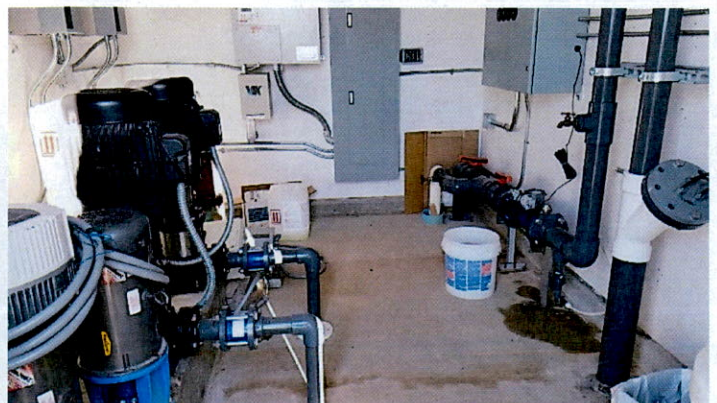
Pump house boosters and appurtenances
