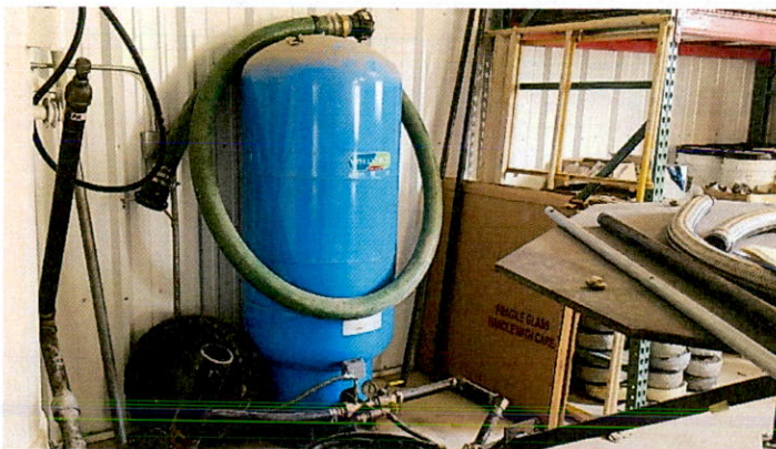
pressure tank installation inside double garage
