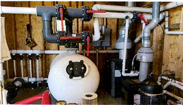
Sand filter and heaters for pool
