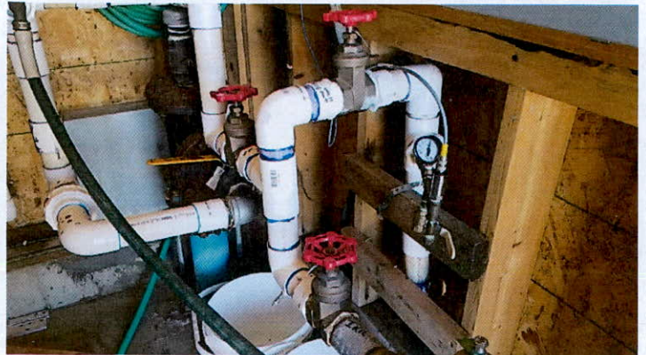
Incoming plumbing – 2" from Madison well (with gauge) City water (backup supply) through 4" line (blue)
