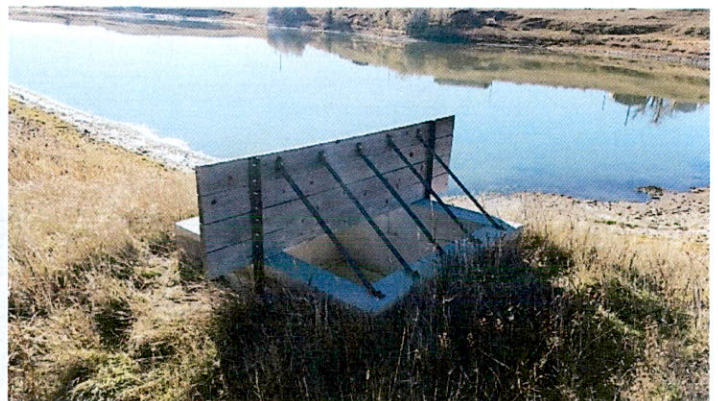
riser and trash rack
