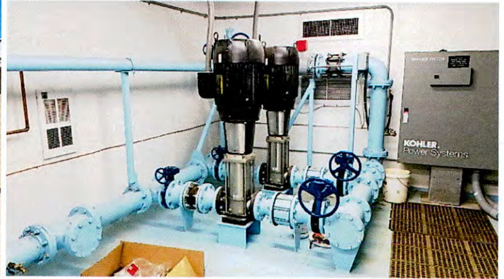
Booster pumps and piping
