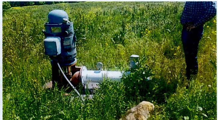
Turbine and air/vac valve
