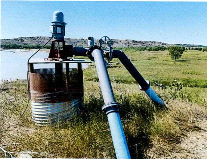
Turbine pump serving both east and west pivots - PVC pipe in foreground is routed to unused center pivot pad
