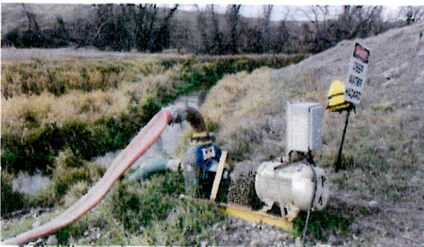
Pump on Redwater Canal 10/19/16
