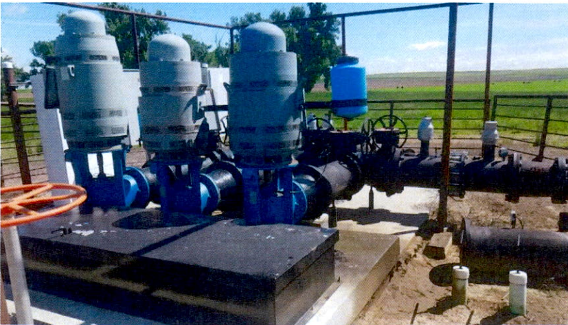
Steel vault in foreground is access location to pumping gallery for 3 turbine pumps serving License No. 910A-1 and the submersible pump serving livestock License No. 1914-1.
