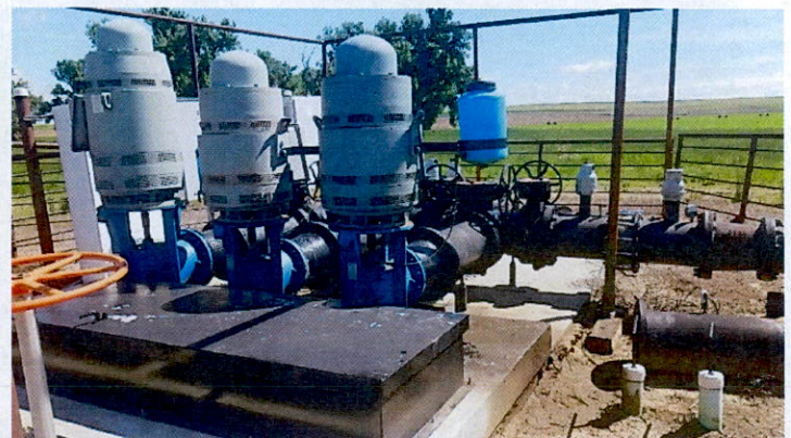
Steel vault in foreground is access location to pumping gallery used for the submersible pump for the livestock system. (also used for irrigation license No. 910A-1)
