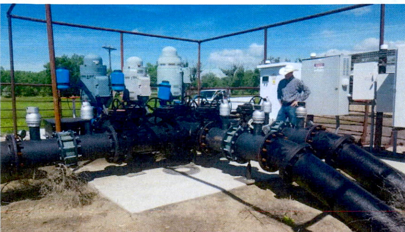
14" steel manifold and valves for sprinkler irrigation License No. 910A-1
