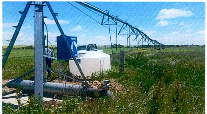
Permit No. 1852-1 pivot and appurtenances
