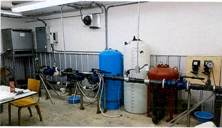
Pump house appurtenances
