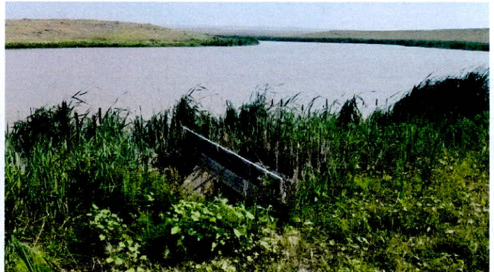
Riser with trash rack and pool
