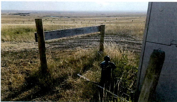
Well and phase converter
